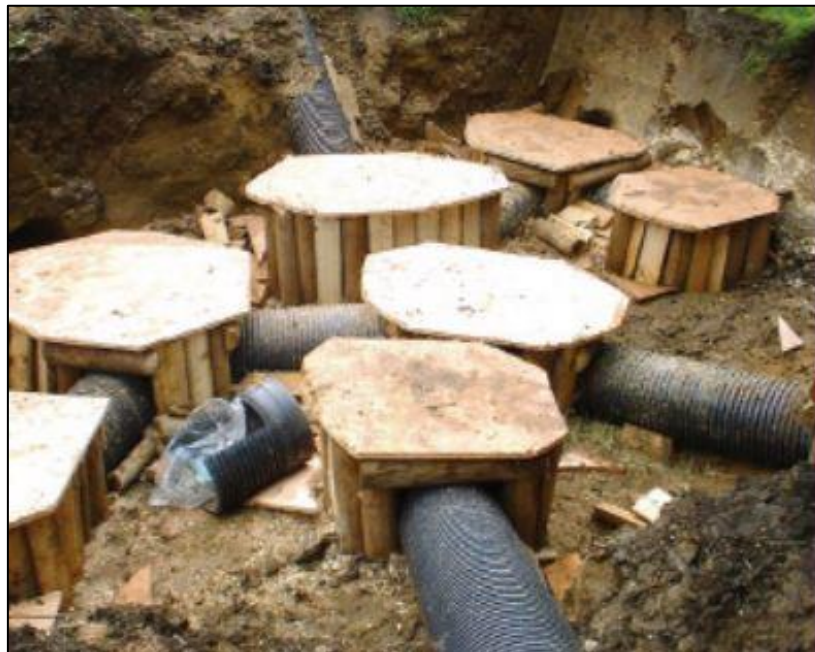
Figure 15-1 An example of an artificial sett under construction with pipe tunnels and 7 chambers (Extracted from NRA (now TII), 2005b)
